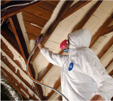
If you don't need much R-value, you can use a two-part DIY spray-foam kit for the foam layer. Be sure to get consistent coverage; this application will need a second layer to fill the cracks.
