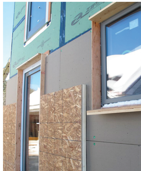
Two layers of polyiso board were added to the exterior of the home, with the seams of each layer of polyiso staggered both vertically and horizontally. The outside polyiso board is manufactured with an OSB nail base.
