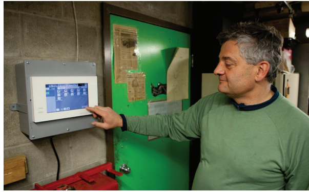
School facilities director Bill Knight shows a visitor the AG-150 touchpad controller for the Mitsubishi heat pump that heats and cools the renovated wing.
