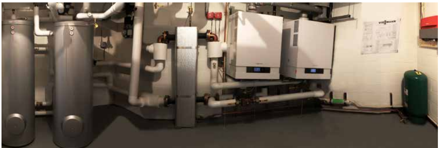
Canterbury's newly spacious boiler room. The dual-coil 79-gallon Viessmann 300-B water tanks (left) can accommodate inputs from solar panels, giving Canterbury the flexibility it wants for future green investments. The Viessmann B2HA 150 condensing boilers (right), compact and easy to service, are surprisingly powerful, producing up to 530 MBH each.
