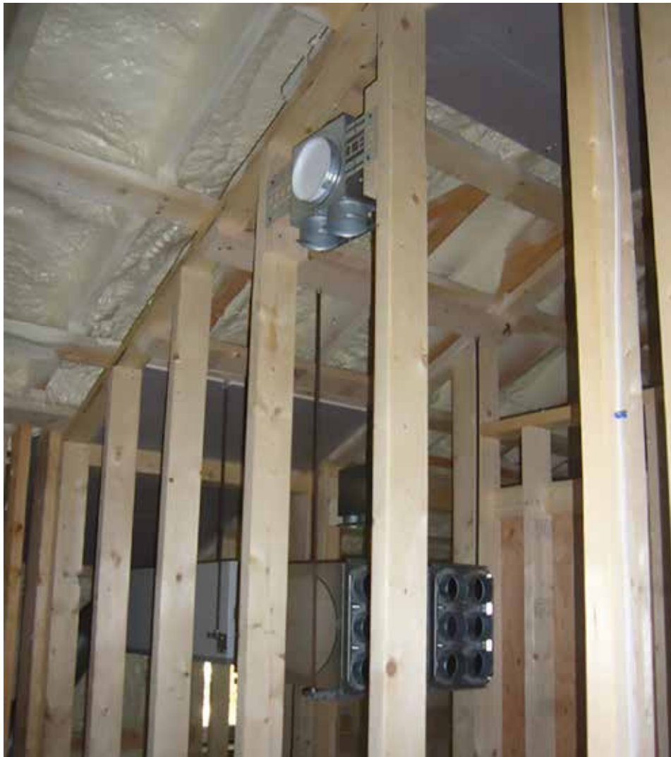
This interior wall and foamed ceiling shows a very high-efficiency European heat recovery ventilator and associated fitting for fresh air supply.
