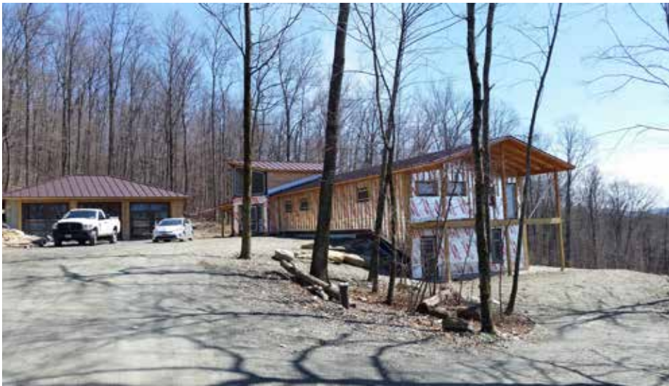
The 8-inch AAC walls are clad with three staggered layers of 1.5-inch polyiso held to the block with a blocking/furring designed by Bruce Coldham. The cumulative R-value of the wall assembly is a true R-40 with zero thermal bridging. Next up: fiber cement siding.
