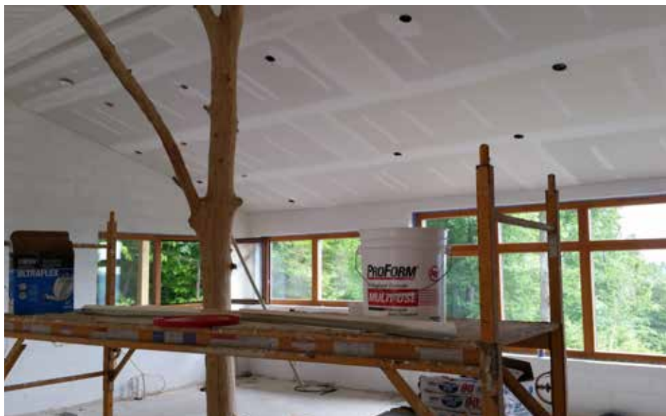
An afterthought to use LED hi-hat light fixtures in most rooms meant the ceilings had to be furred down. The empty space was filled with fiberglass batts, bringing the congregate insulation value of the roof to an average R-65.
