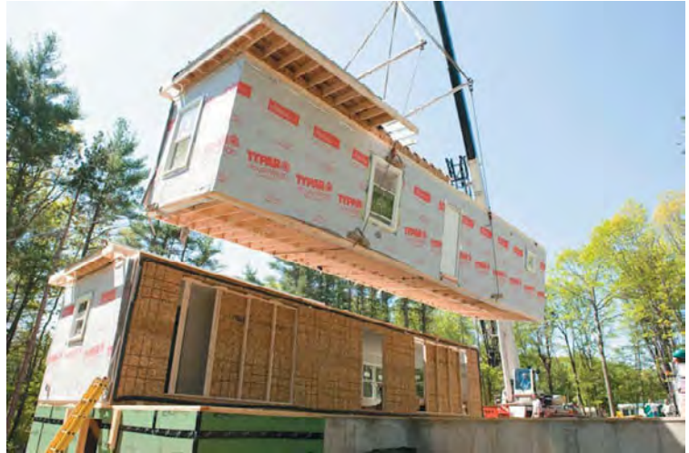
DURING THE CONSTRUCTION PROCESS, BOXES WERE PLACED AT THE FIRST APPLDRE MODEL THAT BRIGHTBUILT HOME CONSTRUCTED IN WELLS, MAINE. (PHOTO TAKEN MAY 24, 2012.)
