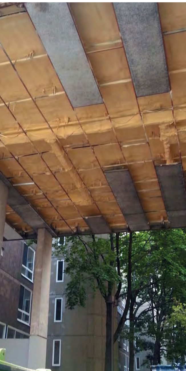
INSULATION IS BEING INSTALLED UNDER AN EXTERIOR FLOOR AT ROOSEVELT LANDINGS. THE PHOTO WAS TAKEN ON JUNE 26, 2013.
