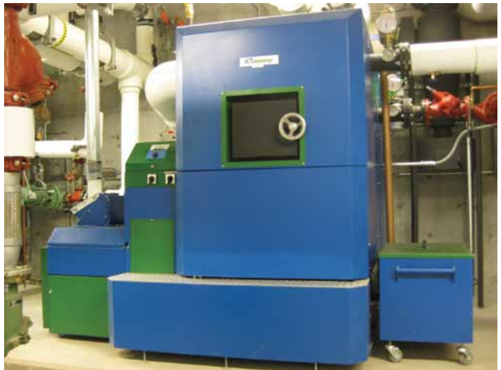
1.7 million Btu per hour boiler supplied by ACT Bioenergy.
