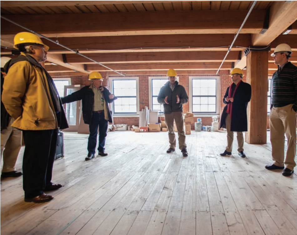
BE13 attendees get an in-progress look at the Fraunhofer Center for Sustainable Energy Systems' renovation and deep energy retrofit of a historic Boston building.
