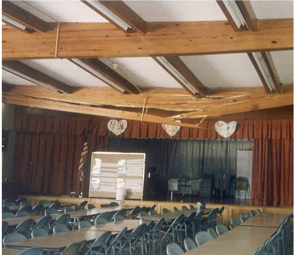
At this New York State elementary school, a 30-year-old beam broke apart following a foot of snowfall. A newly insulated roof had prevented the melting that occurred in the past.
