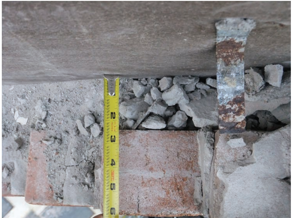
Not good: a rusted brick tie.
