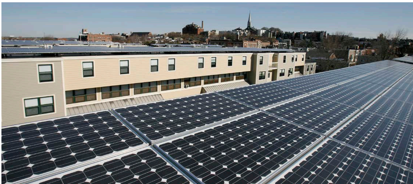
A solar installation on sixteen buildings at Mishaawum Park Apartments in Charlestown, Massachusetts, serves 337 units of affordable housing.
