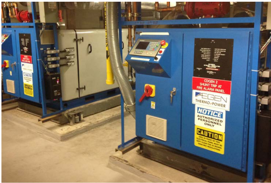
One of two cogeneration units at LB Johnson Apartments in Cambridge, Massachusetts. These units provide heat and domestic hot water while also providing 56% of the electricity used in this high rise elderly housing apartment building.
