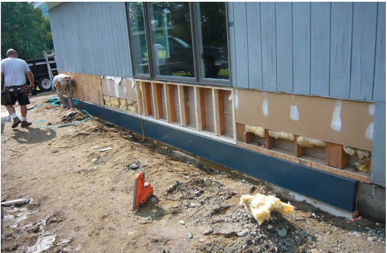
THE EXTERIOR OF PLAINFIELD SCHOOL AT DIFFERENT PHASES OF THE TRANSITION, AS IT UNDERWENT ITS DEEP ENERGY RETROFIT. PHOTO CREDIT: MARC ROSENBAUM.
