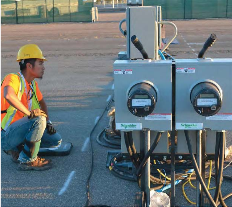
A SOLAR DECATHLON TEAM MEMBER SURVEYS MICROGRID EQUIPMENT THAT WILL BE USED TO POWER THEIR HOUSE. PHOTO CREDIT: AMY VAUGHN/U.S. DEPARTMENT OF ENERGY.
