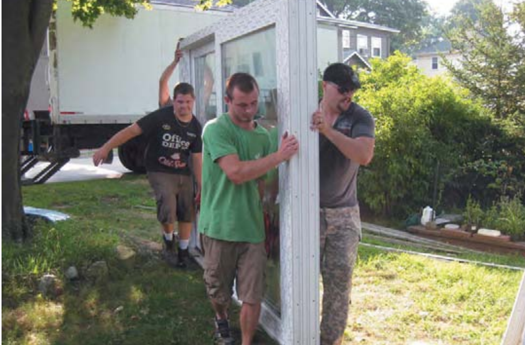
A WORK CREW DELIVERS A HIGH-EFFICIENCY WINDOW TO BE INSTALLED IN A RESIDENTIAL DEEP ENERGY RETROFIT PROJECT IN UPSTATE NEW YORK. PHOTO CREDIT: US DEPT. OF ENERGY.
