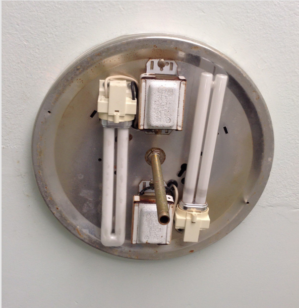
Typical (used) CFL “pan” fixture shown w/out diffuser; 2 13W twin tubes
