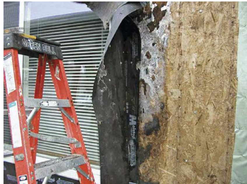
JLC, George Tsongas, Sheathing Damage From Using Wide Impermeable Flashing
