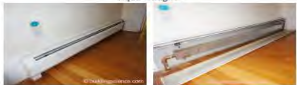
Photograph 1a (left): Baseboard Radiator; Photograph 1b (right): Liquid Gas Heat Exchanger
