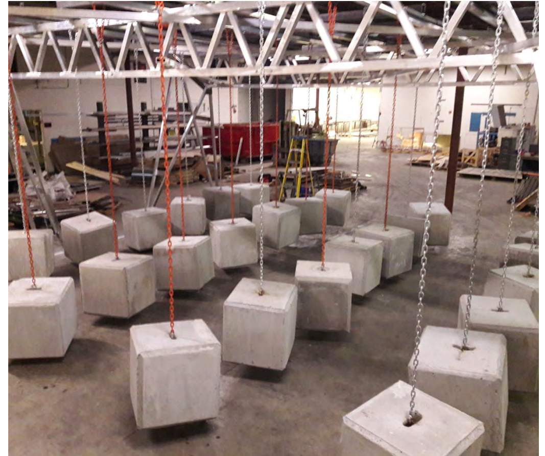
Maley Laser manufacturing facility Warwick, R.I., 2018
