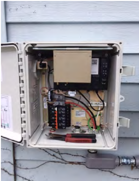
Combiner box containing the modem and breakers
