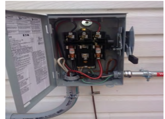
AC Disconnect containing Overcurrent Protection Device
