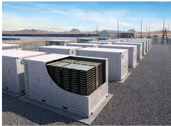
Battery energy storage
