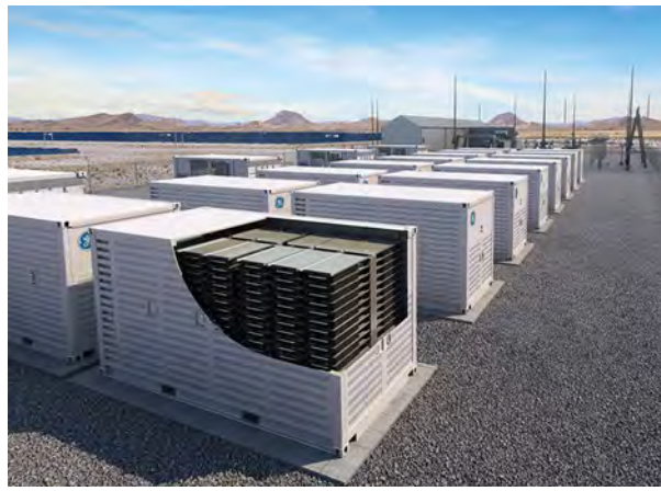
Battery energy storage
