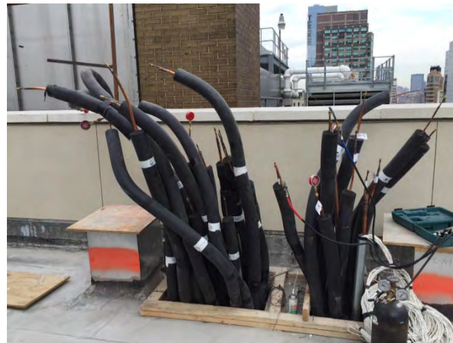
REFRIGERANT PIPING ON ROOF
