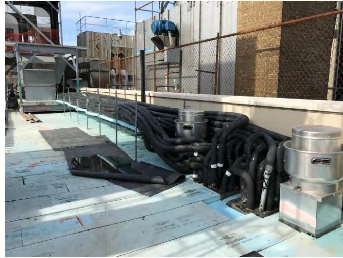
REFRIGERANT PIPING ON ROOF
