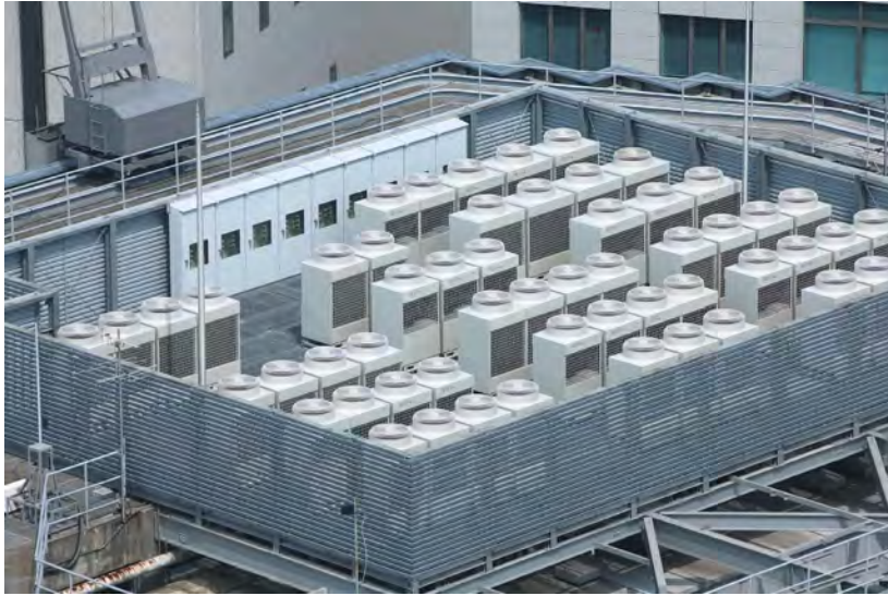
CONDENSER "FARM" ON ROOF
