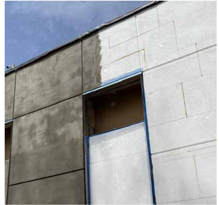
Above grade: 5" EPS continuous exterior insulation added R-19 to the existing mass walls Below grade: R-15 (down 12")
