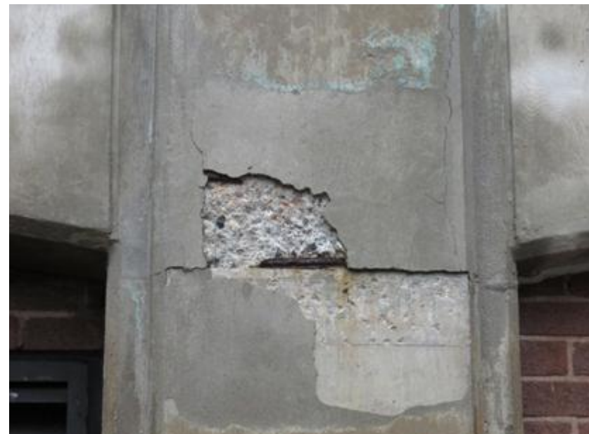
FAILED CONCRETE PATCHES
