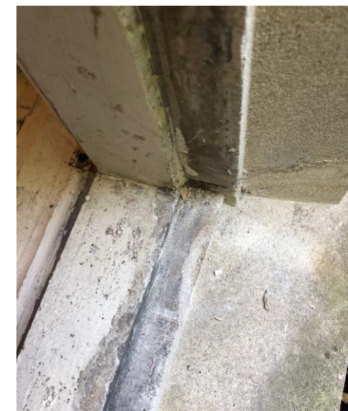
WINDOW SILL CONDITION
