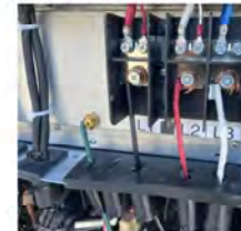
Close-up photo of wiring:
