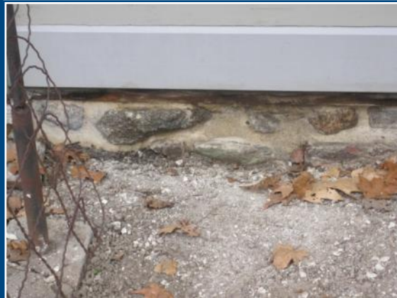
Holes in Foundation
