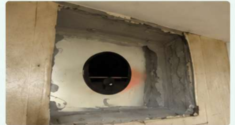
Exhaust Register (After)
