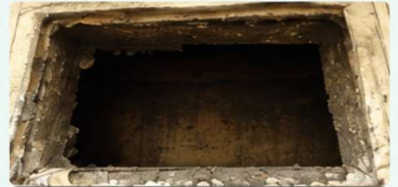
Exhaust Register (Before)
