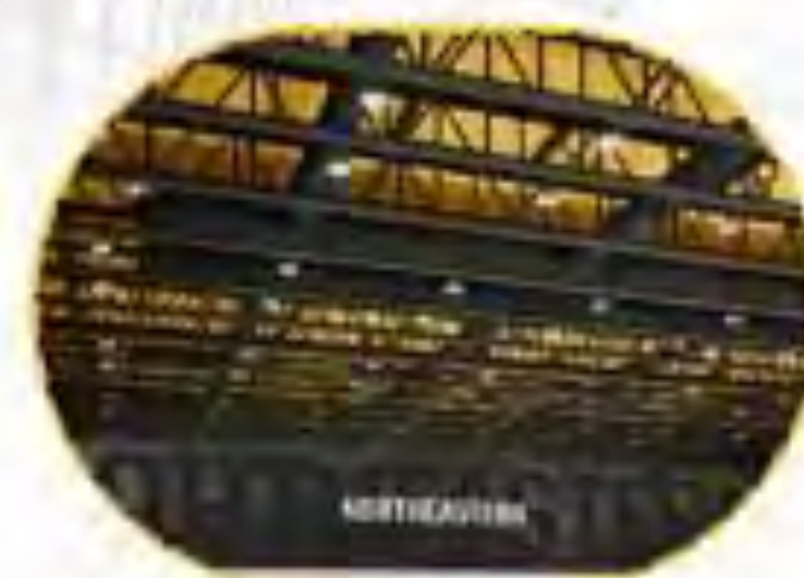
Cross Laminated Timber Roof
