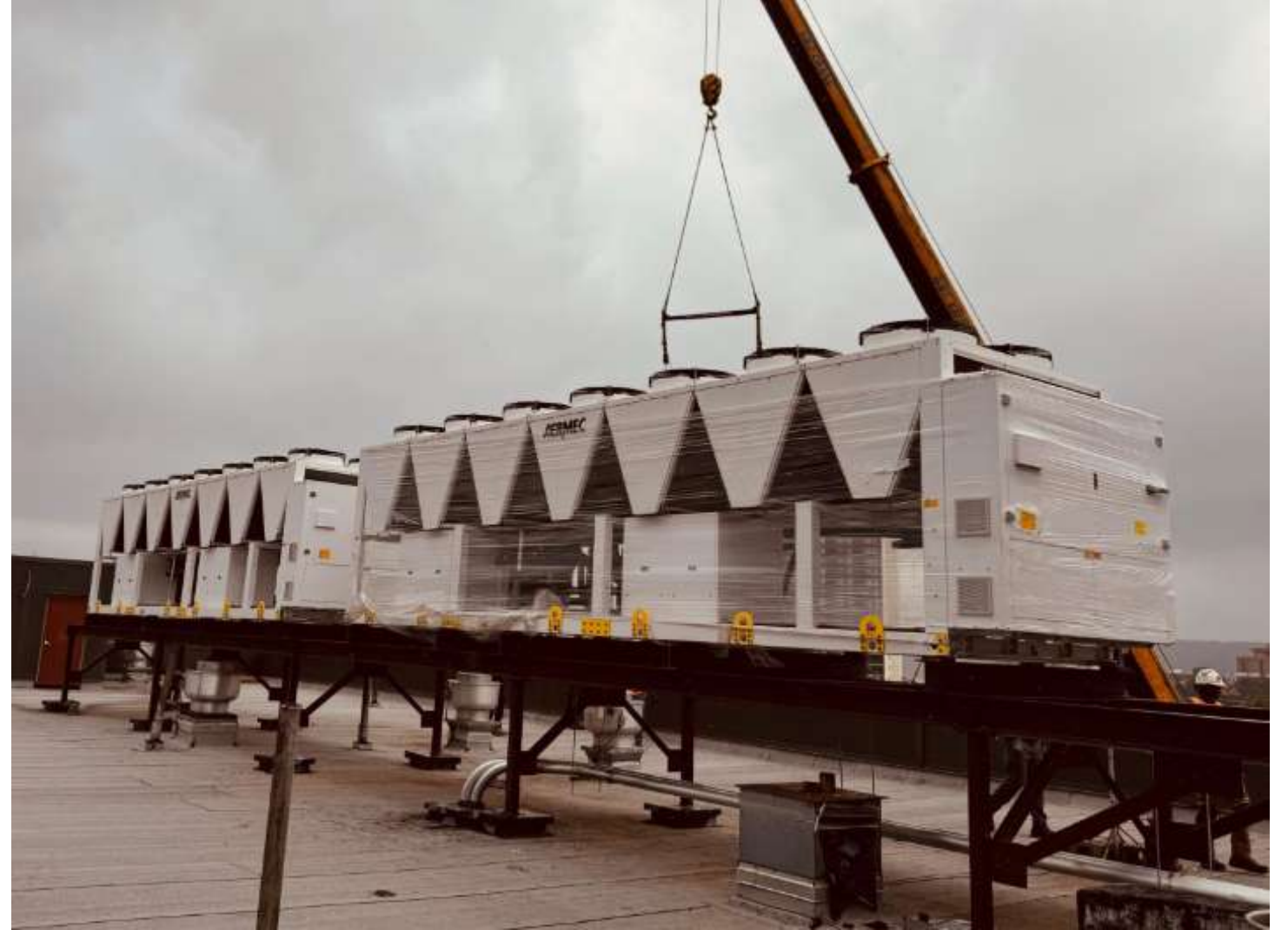
Rooftop Heat pump
