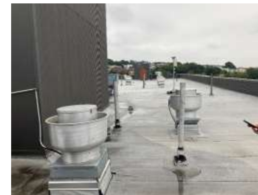
Rooftop exhaust fans
