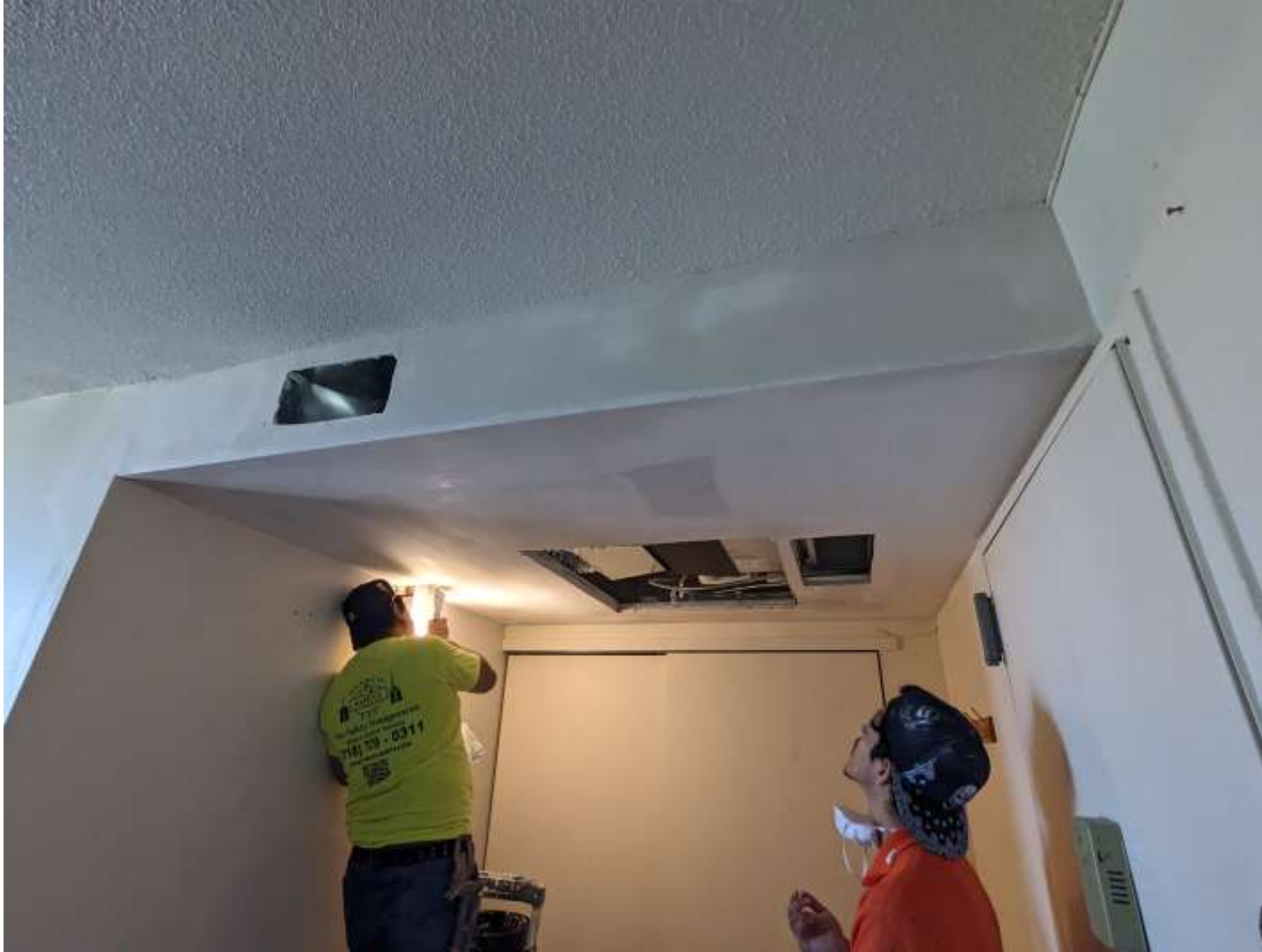
Terminal unit at entry
