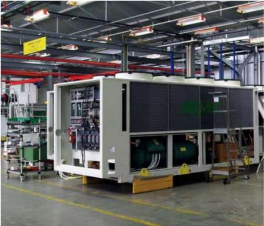
Aermec NYK modular air-to-water heat pump – basis of design, 9 modules (~200 tons) per tower
