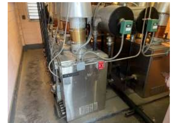
Gas DHW plant (modular boilers)
