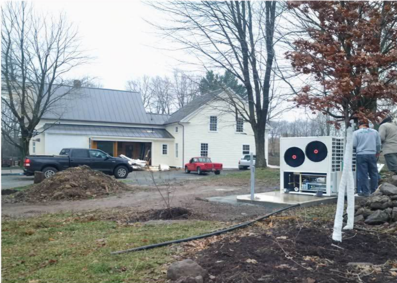
Example: Remote installation serving a residential hydronic system
