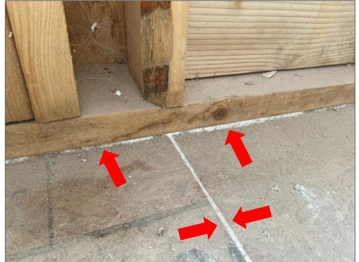
Sealant at Base Plate & Subfloor of 3 rd Floor (AeroBarrier still found & sealed leakage where caulk was installed)
